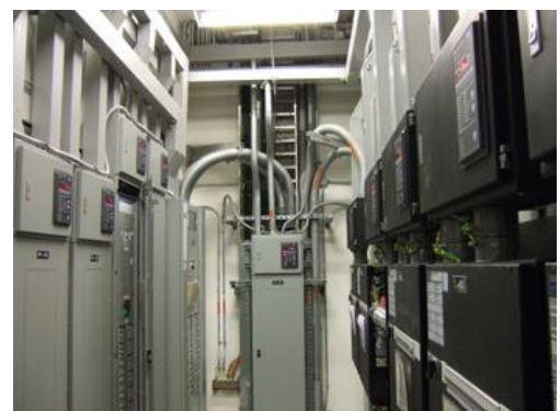
Lutron Lighting Panels interfacing to FieldServer
